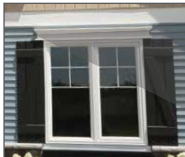
Crosshead too long
